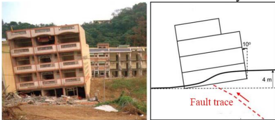
Figure 1. Analysis Diagram of Structural Failure on Fault Traces
