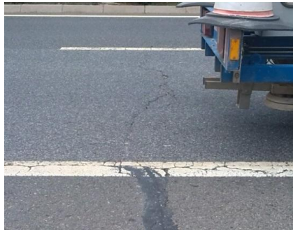
1) Crack Field Test
