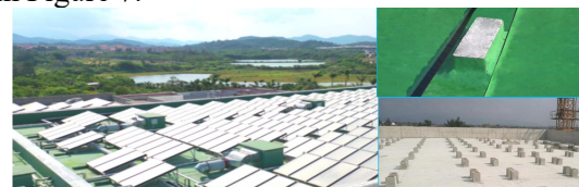
Figure 6. Solar Panel Support Piers for the Project
