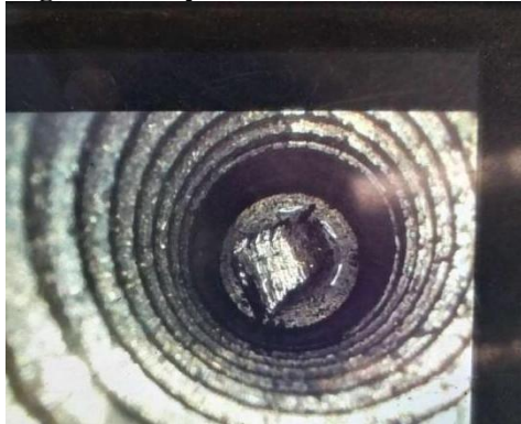
Figure 5. Iron Filings in the Bolt Holes
