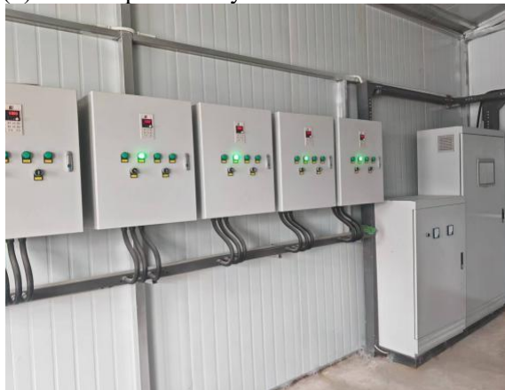
Figure 3. Control Cabinet Data Acquisition System
